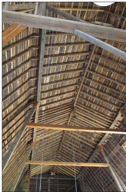
LOOKING UP: The voluminous ceiling inside the barn has a complex post-and-beam structure that supports the barn.
